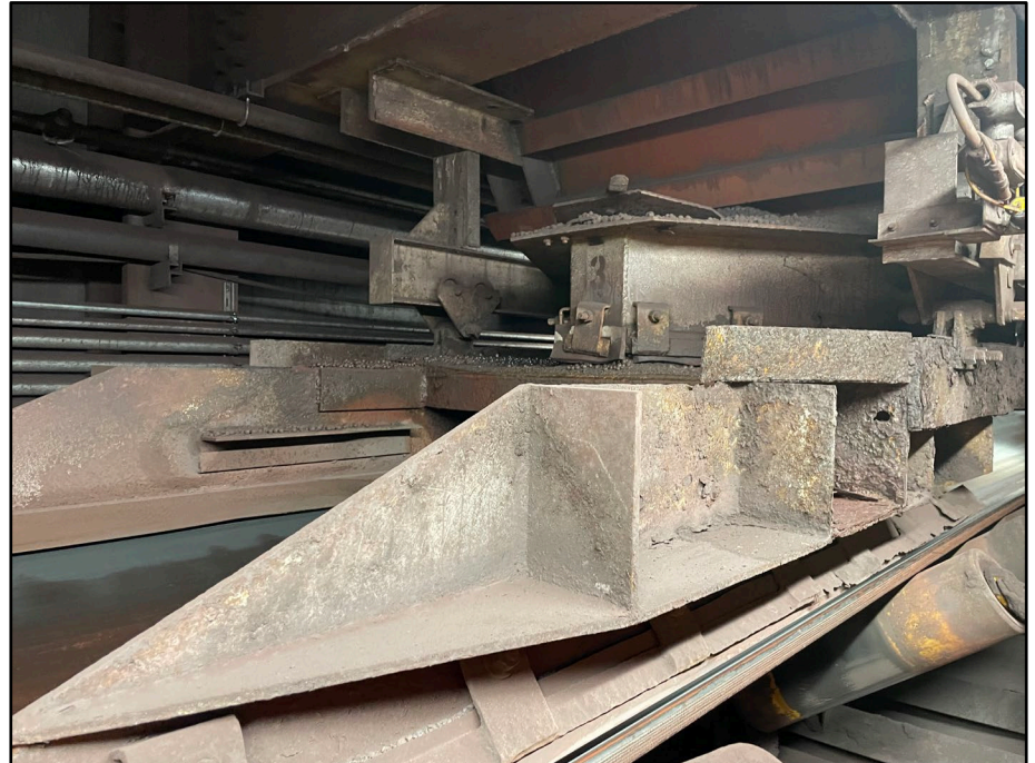
Example conveyor system hopper
